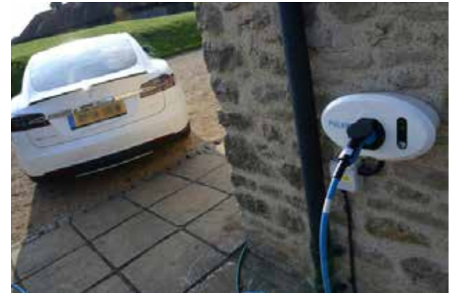
F.35 Example of on-plot EV charging point (elsewhere in the UK).
