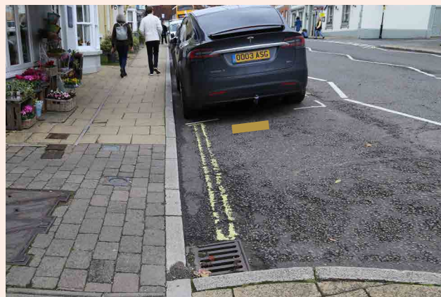
Figure 53: Inadequate drainage strategy on West Street.
